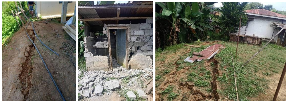
Earthquake damages to houses and lands in Tamac, Villaviciosa, Abra
