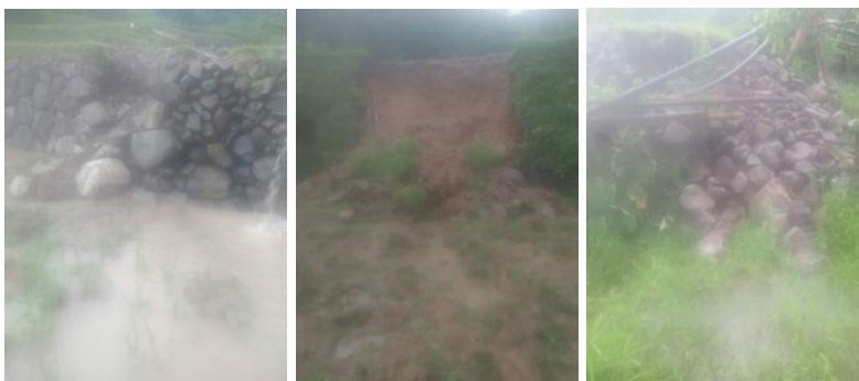
Earthquake damages to a rice field in Bazar, Sallapadan, Abra
