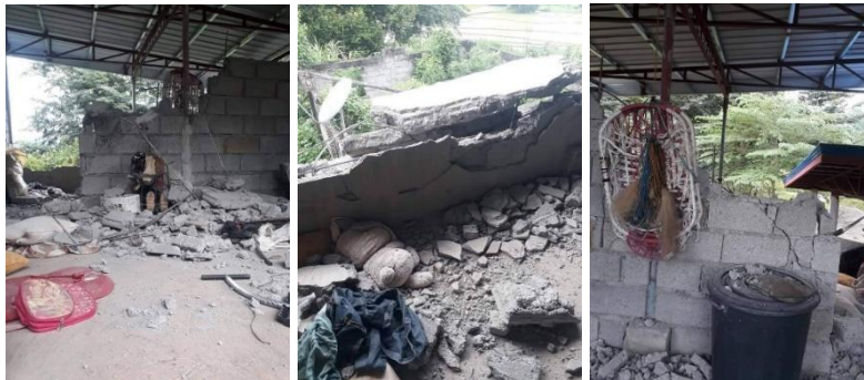
Earthquake damages to a house in Tubo, Abra
