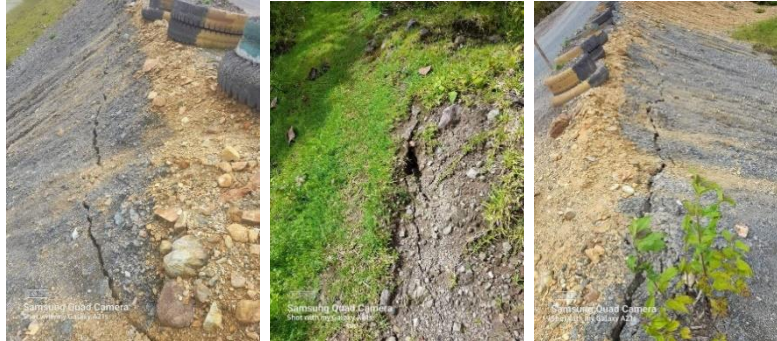
Lepanto Tailings Dam 5-A (located upstream of Abra) after the 7.0 magnitude earthquake
